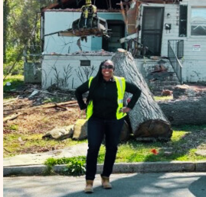
Dee Jordan, Founder & CEO of Jordan Home Builders LLC, stands proudly in front of a demo project in East Durham, showcasing her dedication to revitalizing communities in partnership with DCLT.
