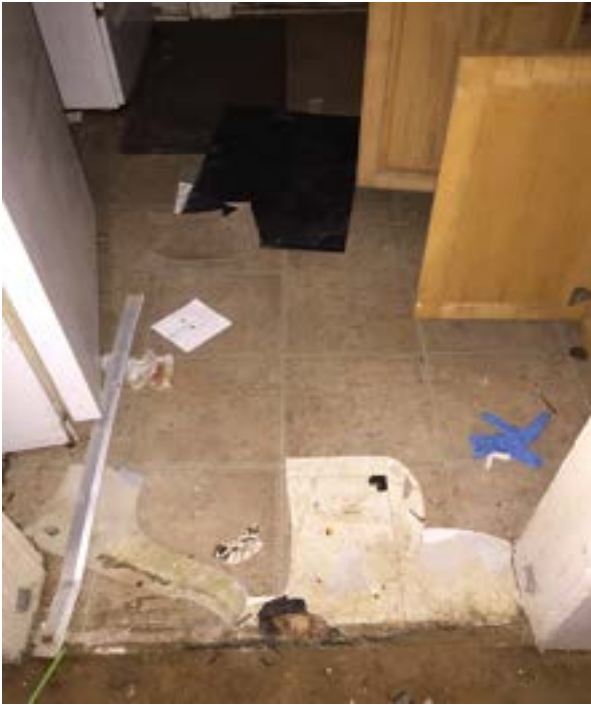
PHOTO No. 5 Typical View of 1106 Alma Street Kitchen Flooring with Multiple Floor Coverings
